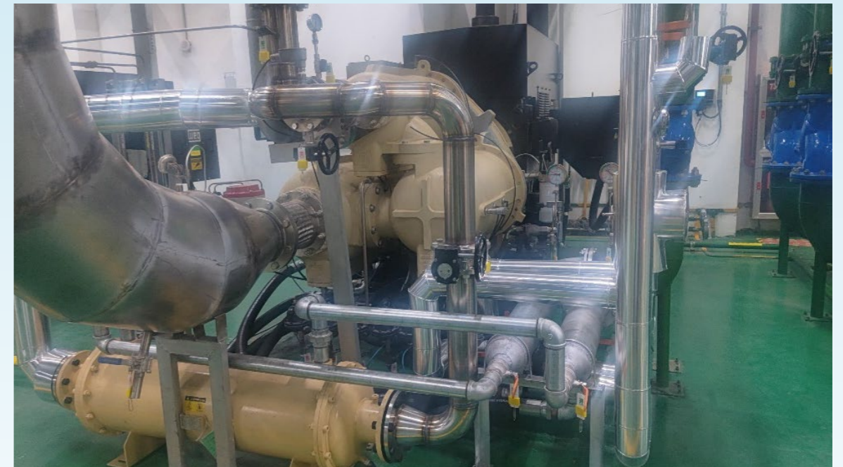
Heat Transport Pipelines
