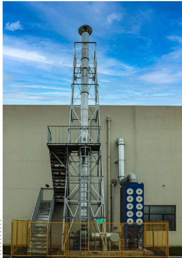
Waste Gas Treatment Facilities
