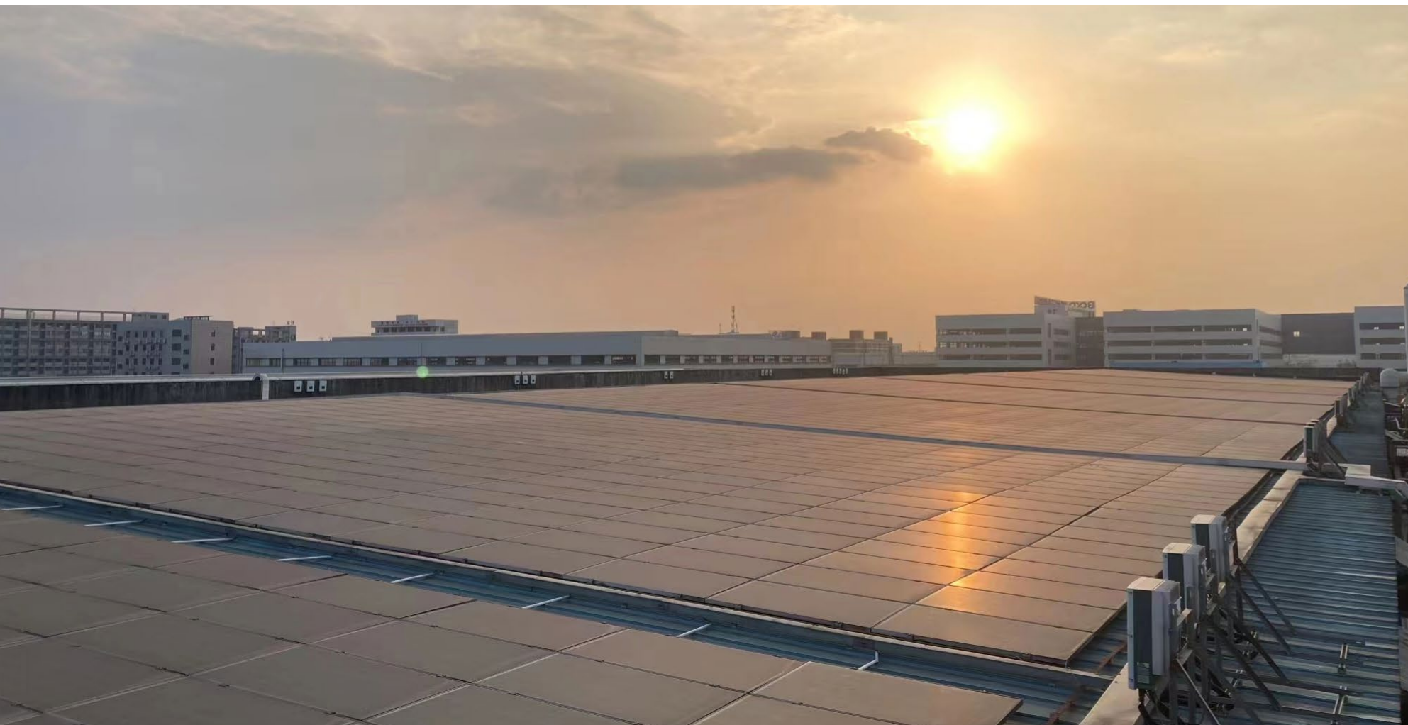
Foshan Base PV Generation Project on Rooftops
