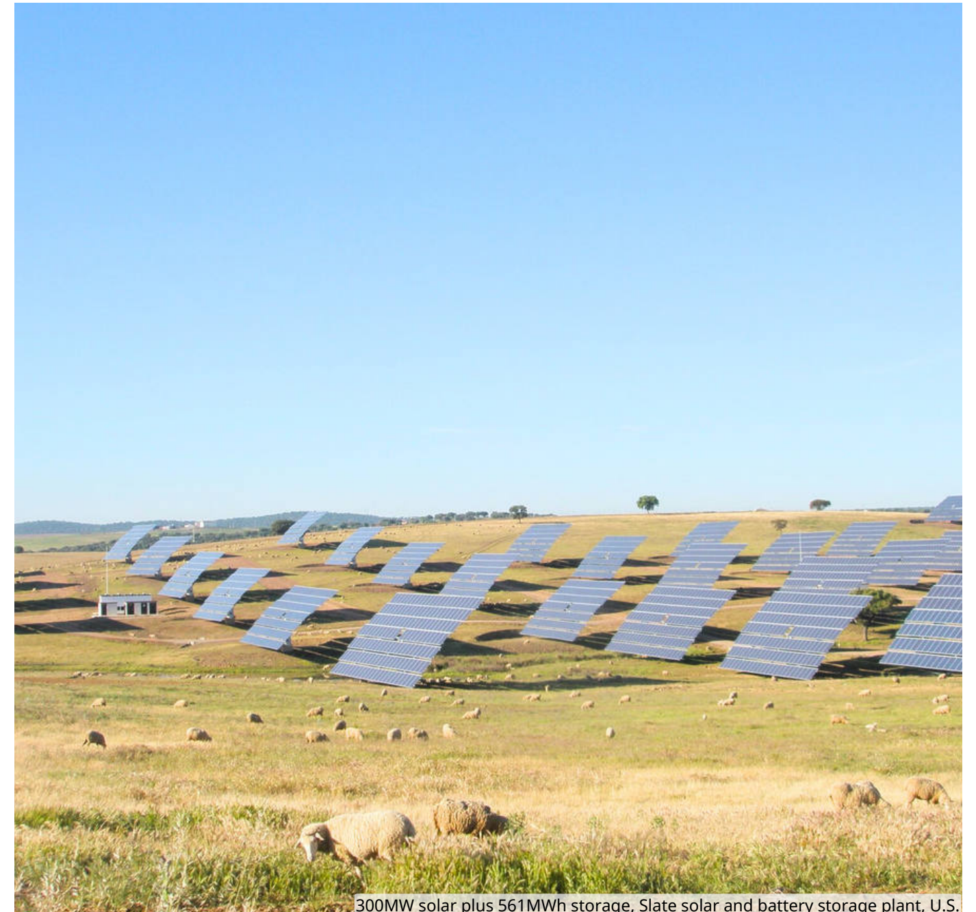
300MW solar plus 561MWh storage, Slate solar and battery storage plant, U.S.
