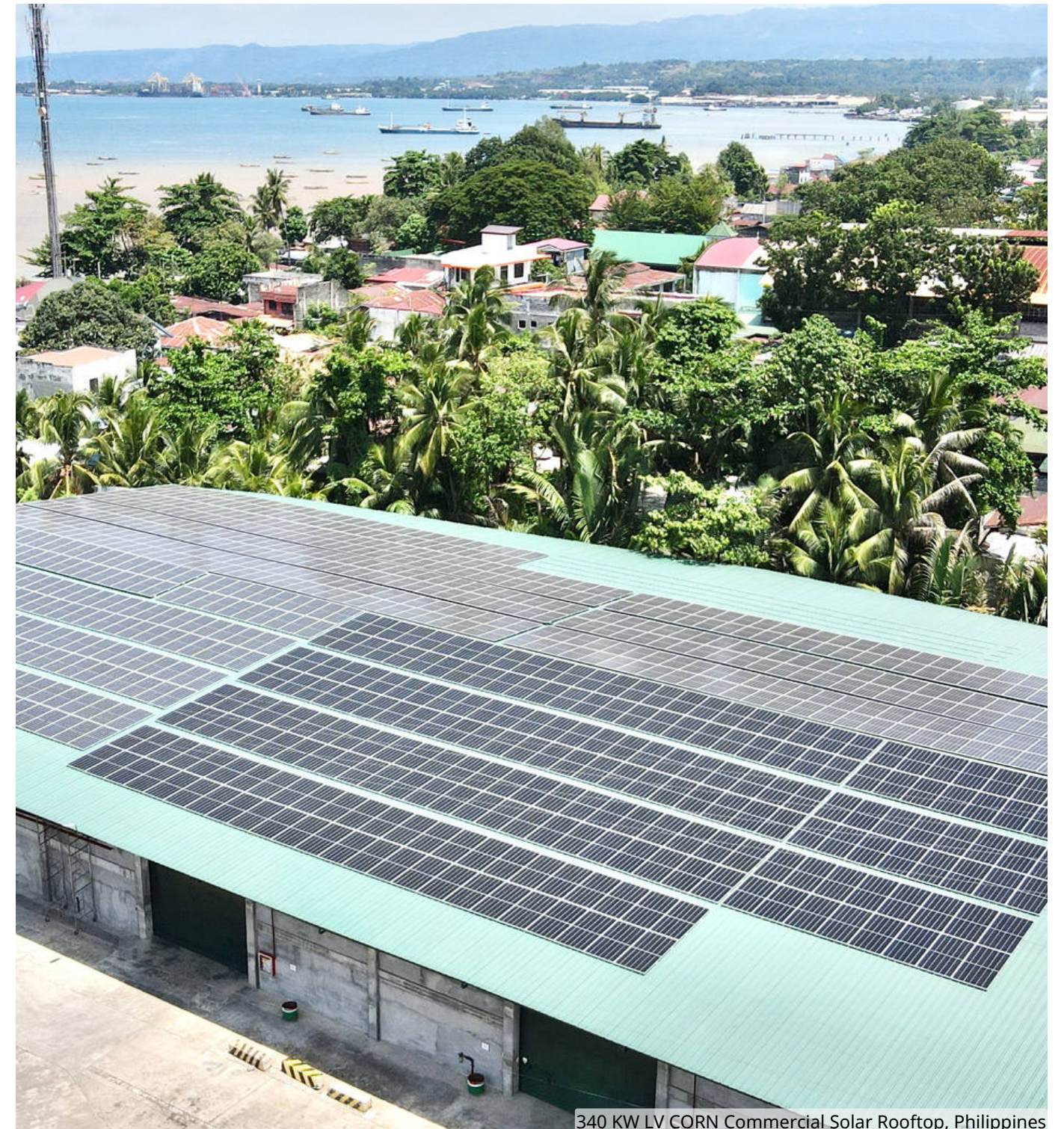
340 KW LV CORN Commercial Solar Rooftop, Philippines
